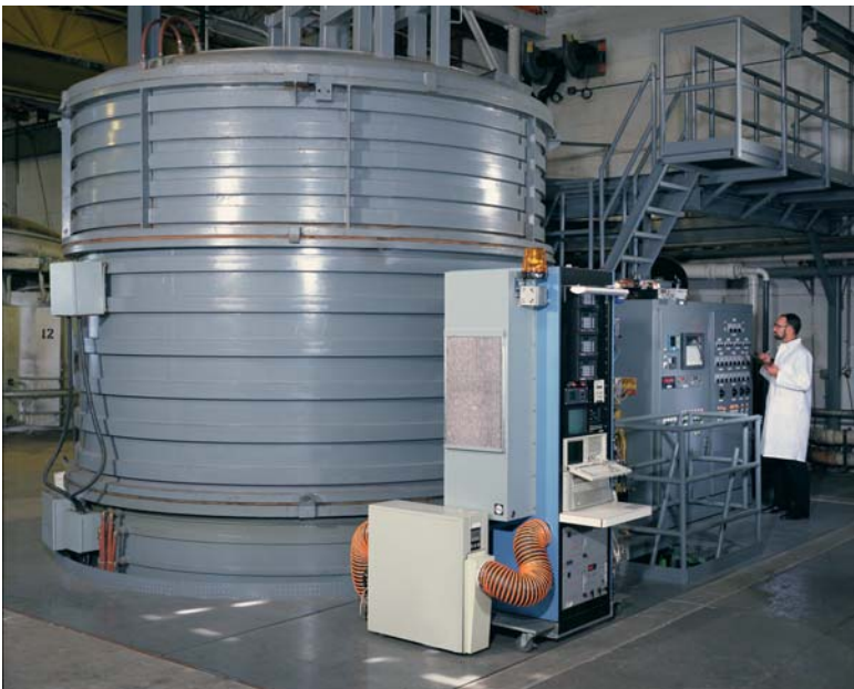
The world's largest commercial top-loading vacuum furnace at our processing facility in Dayton, Ohio.
